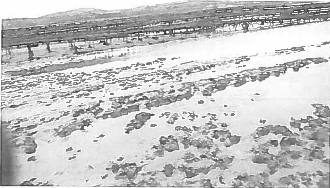
View of soft ground at west end of site 530A – trestles in view are on site [REDACTED]
